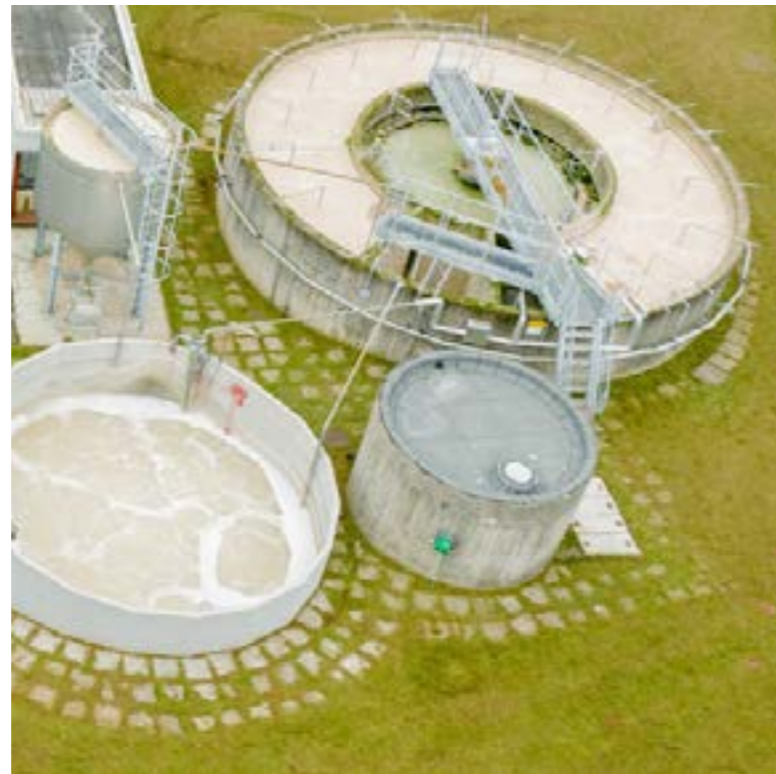
Wastewater treatment plant Origgio Site
