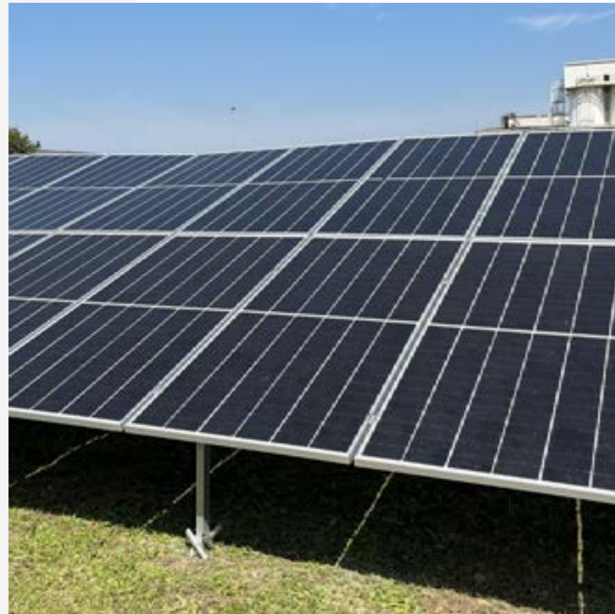
Solar park at Grüenthal's manufacturing site in Origgio
